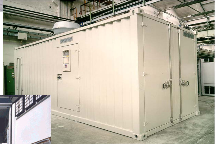
Air-cooled arrangement in container
