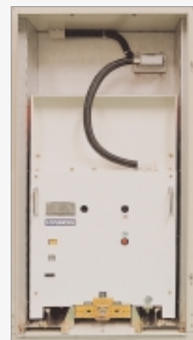
Circuit-breaker in the 'Service' Position
