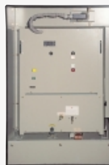
Circuit-breaker in the 'Service' Position
