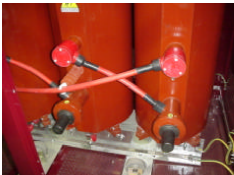
Figure 5 Bushing for HV terminals
